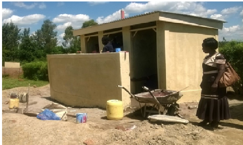
The contractor doing the final works on the sanitation block (two pit latrines and one bathroom)
