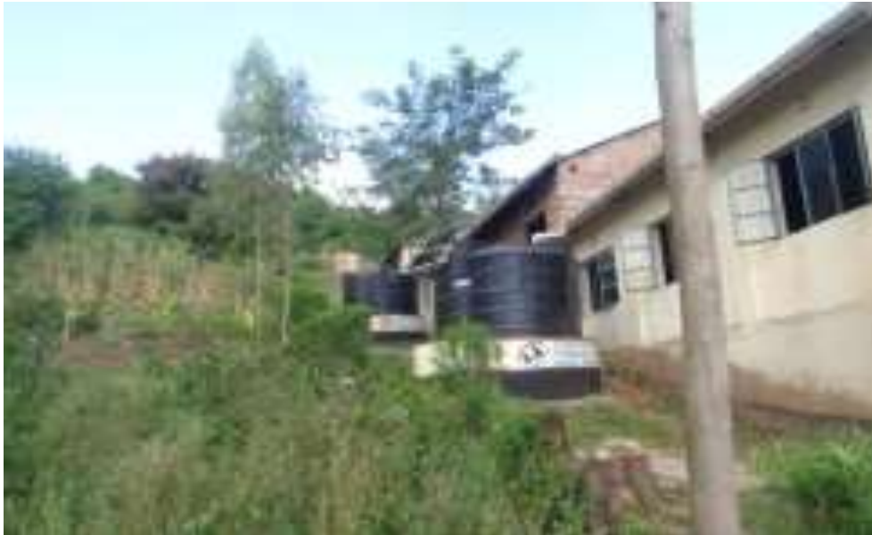
2 Tanks installed at the back of the classrooms
