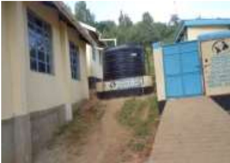
1 Tank installed for use at the sanitary block
