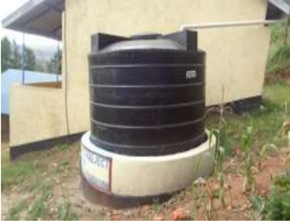
1 tank installed at the side of the classrooms with a tap inform for drawing water
