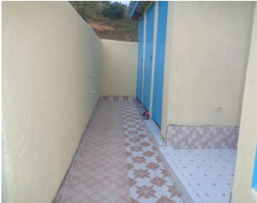
Inside view of the Sanitary Block, Consists of 2 latrines, 1 bathroom and 1 urinal for girls.
